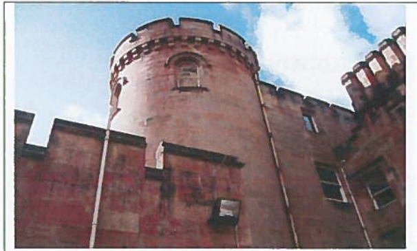
Tower showing Cracking
